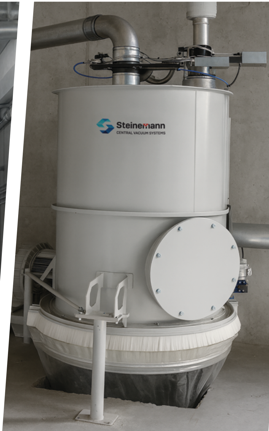
Installed at tripod (short type)
